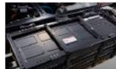
BATTERY 3 72 kWh (3 x 24 kWh each)
